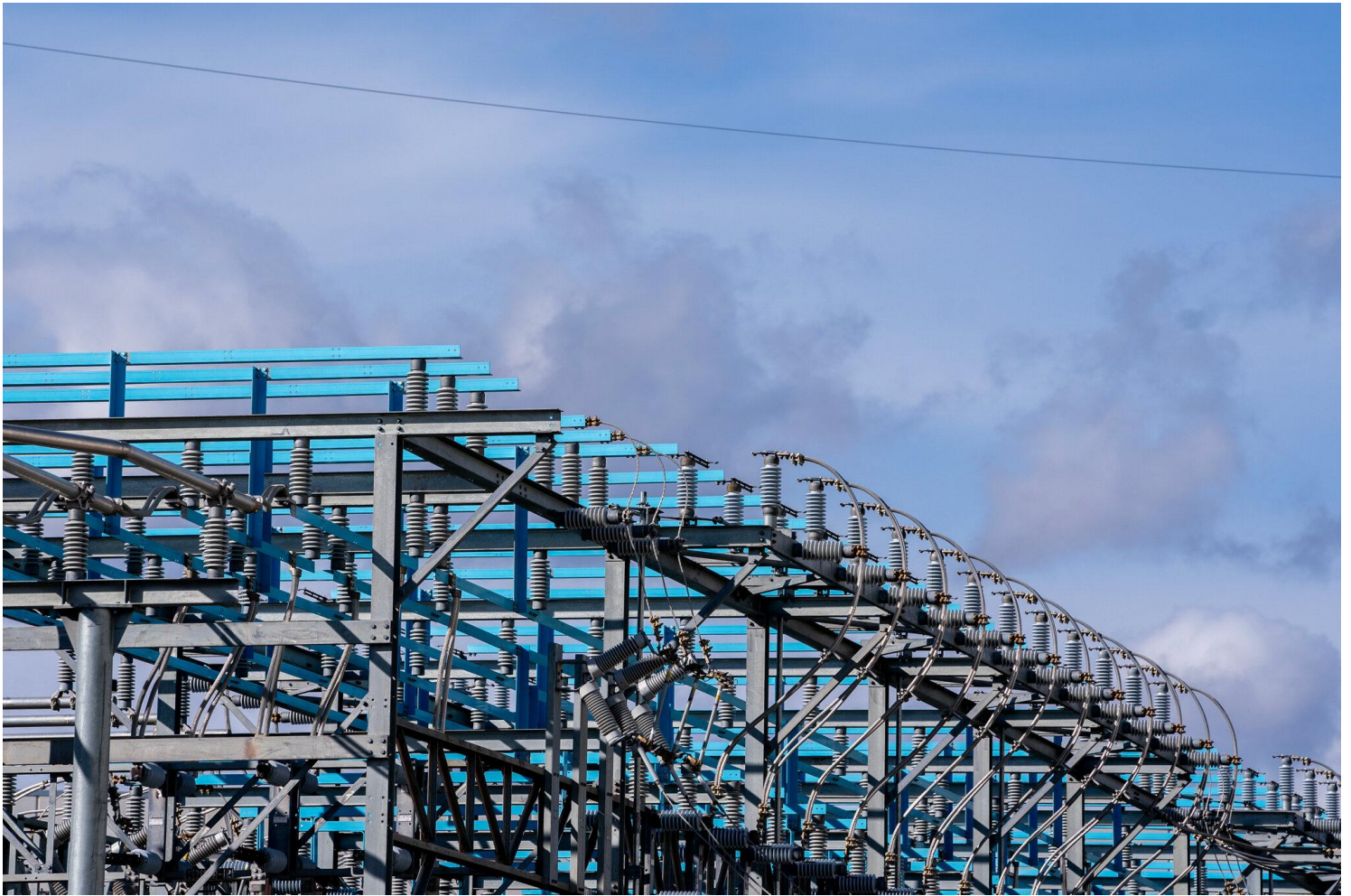
A power substation near a CloudHQ data center in Ashburn, Va. Nathan Howard for The New York Times
